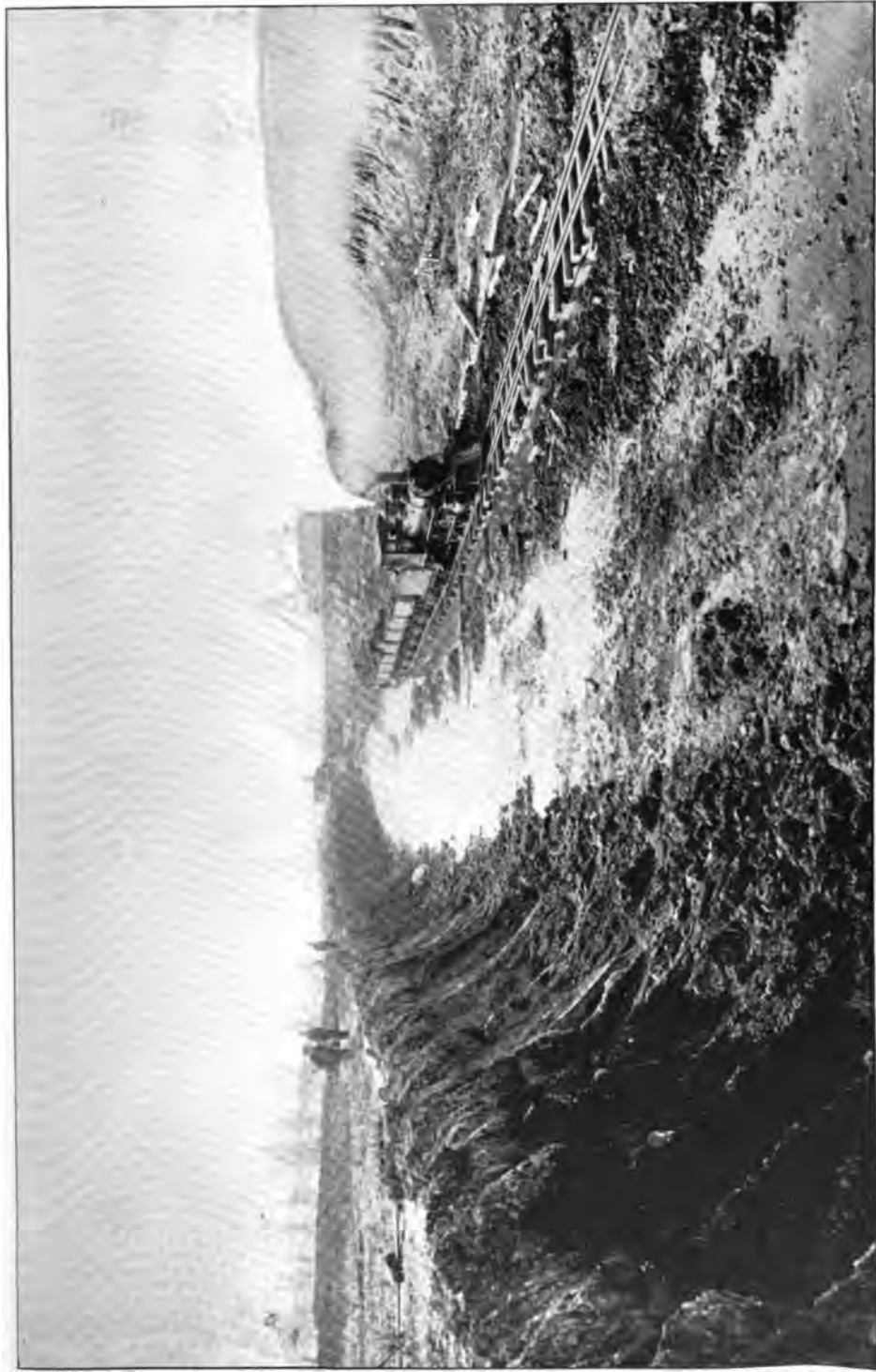
EXCAVATION IN EARTH FOR DRAINAGE CHANNEL AND WATERWAY. ONE THIRD REQUIRED DEPTH.
